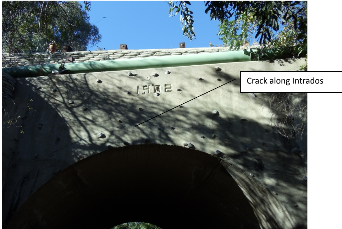
5 Spalls on Wall of Culvert (Southwest Corner)
